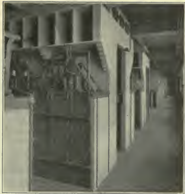
FIG. 491. POWER STATIONS. Circuit Breakers and Compartment, Power Station of the Pennsylvania Railroad at New York City.
